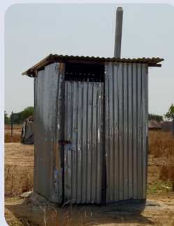
The old toilets were damaged...
